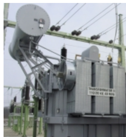
Energetski transformator 110/20 kV moči 40MVA
