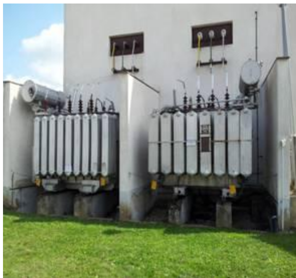
Energetski transformator v RTP Ljutomer
